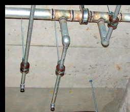
Fire Sprinkler Systems
